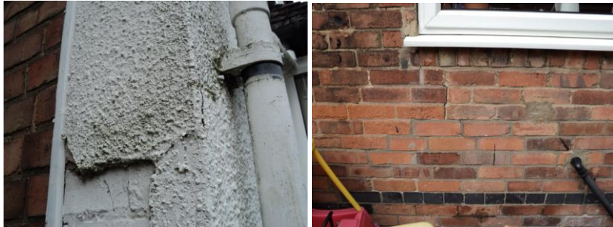
Damaged render to front
