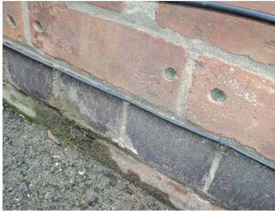
Chemical and blue brick DPC
