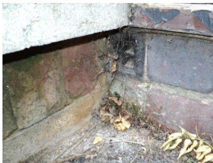
Blocked vent by rear step
