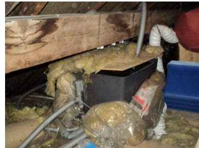
Old stains to rear purlin
